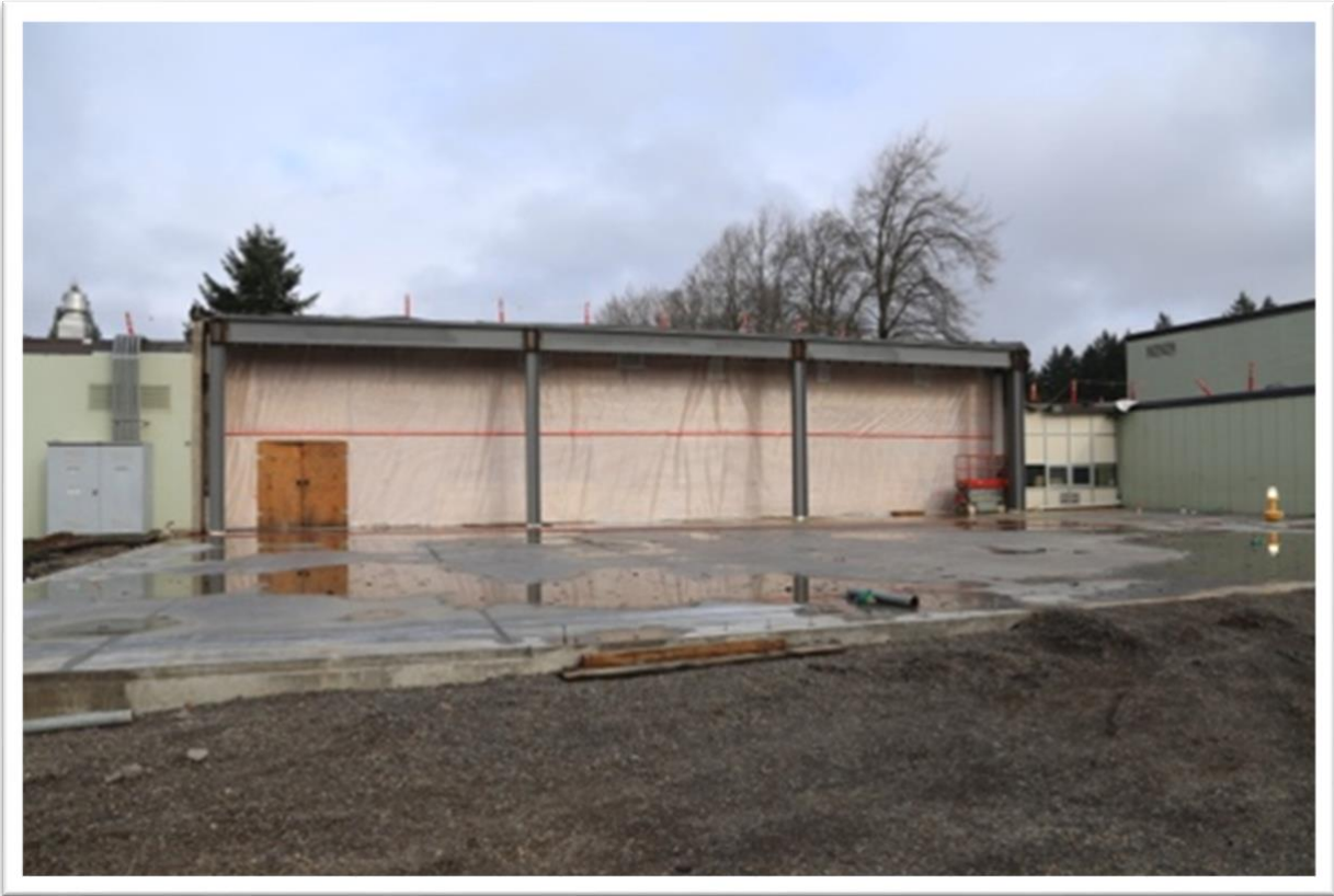
The cafeteria expansion will be built on top of this foundational concrete slab
